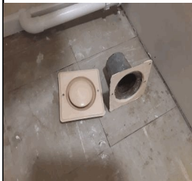
bathroom grill and ducting
