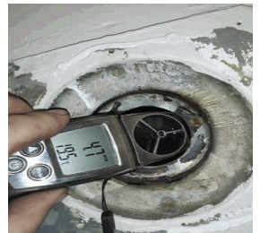
toilet airflow after
