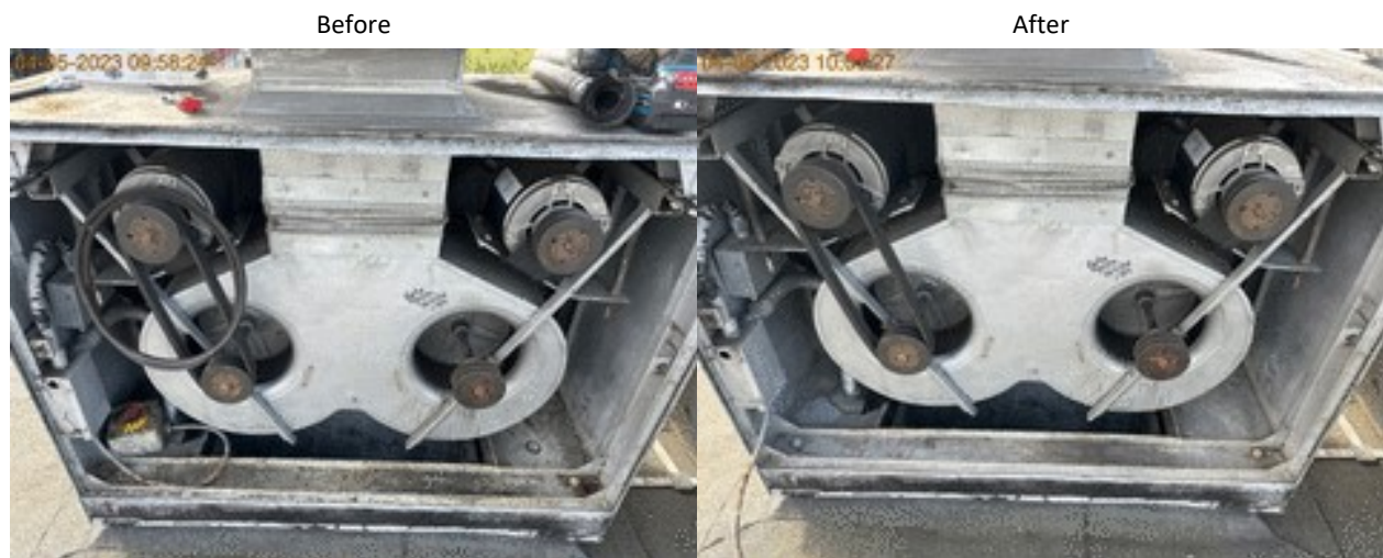
Goulden House - Phase B Fan No.685 far side flats near entrance B - belts changed due to breakage – Extract
