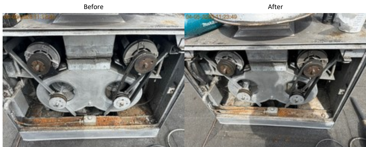
Goulden House - Phase B Flats right hand side 4th floor Fan No.686/687 – Extract
