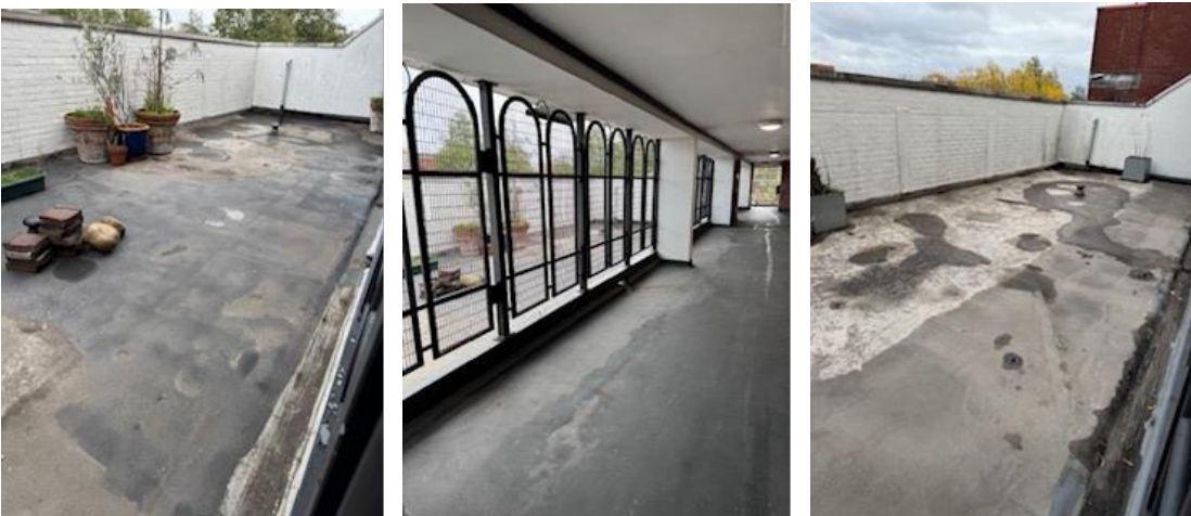
A sample of the photos from the 4 th Floor Terraces after the removal of the stones & pebbles
